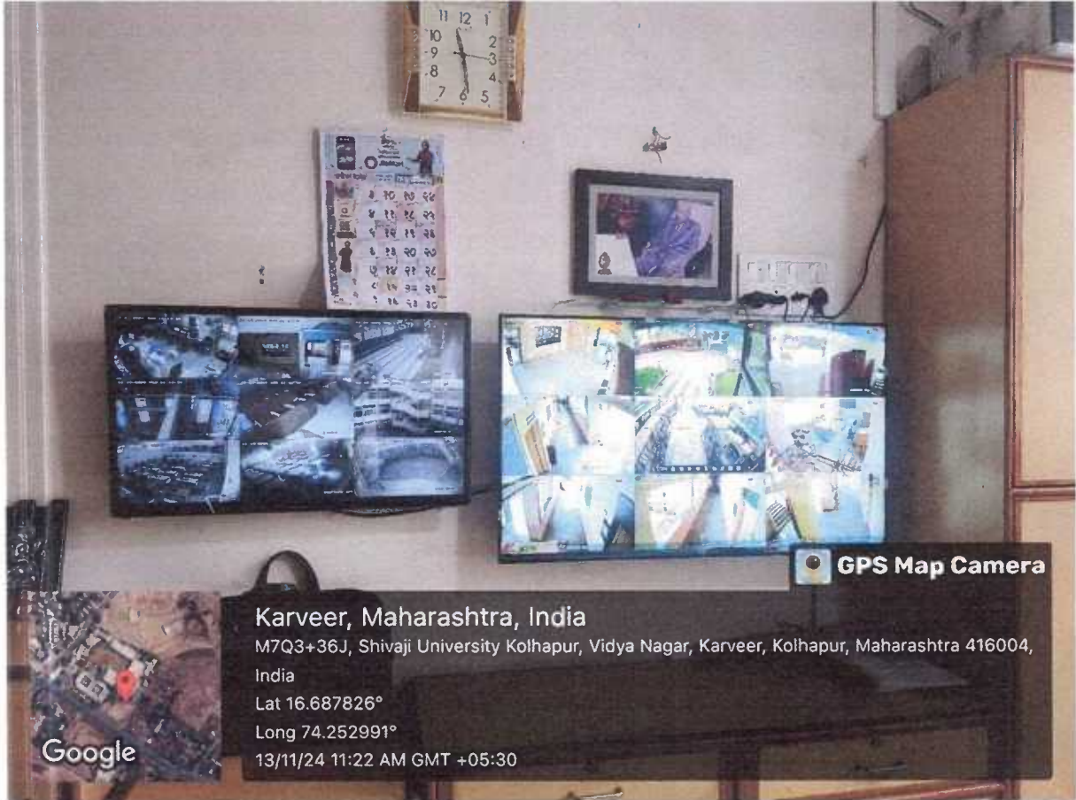
CCTV Mosaic display at Principal's Cabin
