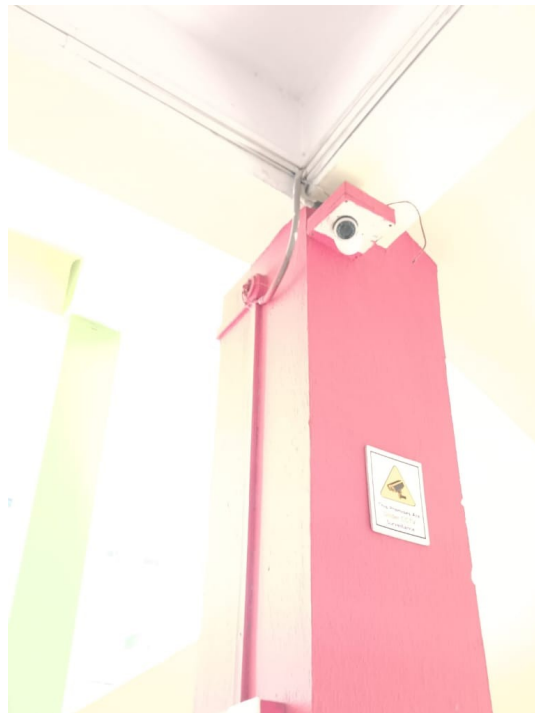
CCTV- Stair Case and entrance
